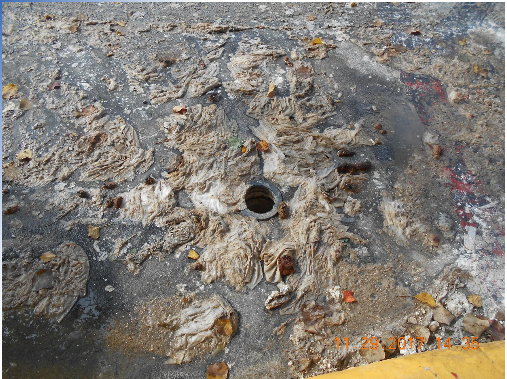
Another open cleanout.
