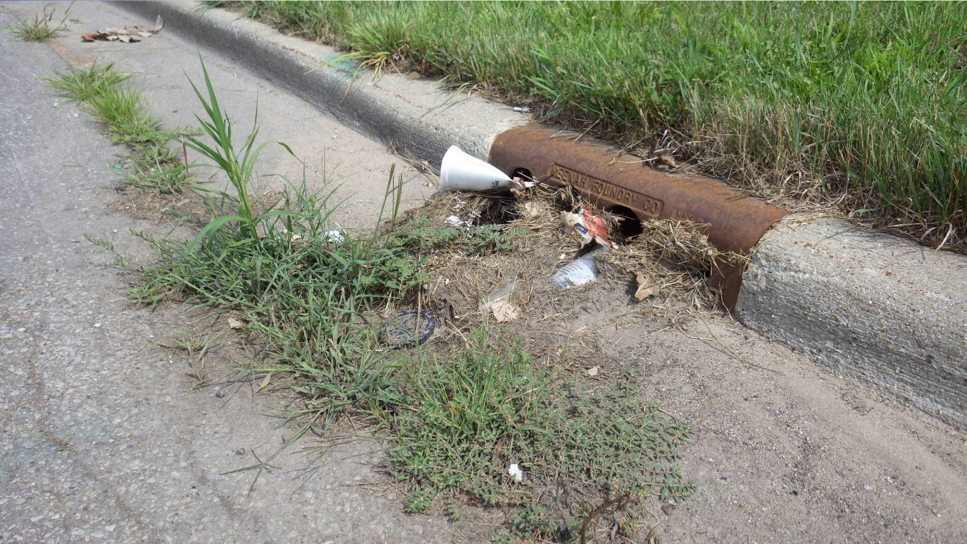
Storm drain clogged with lawn clippings and litter.
