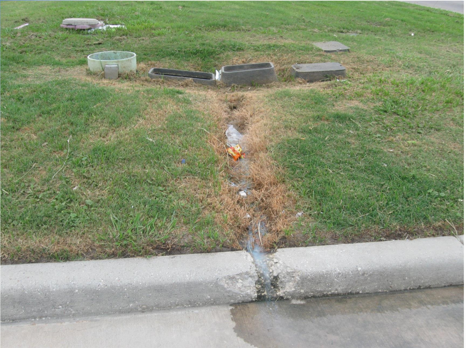
Discharge of sewage and cleaning chemicals from commercial establishment septic system.
