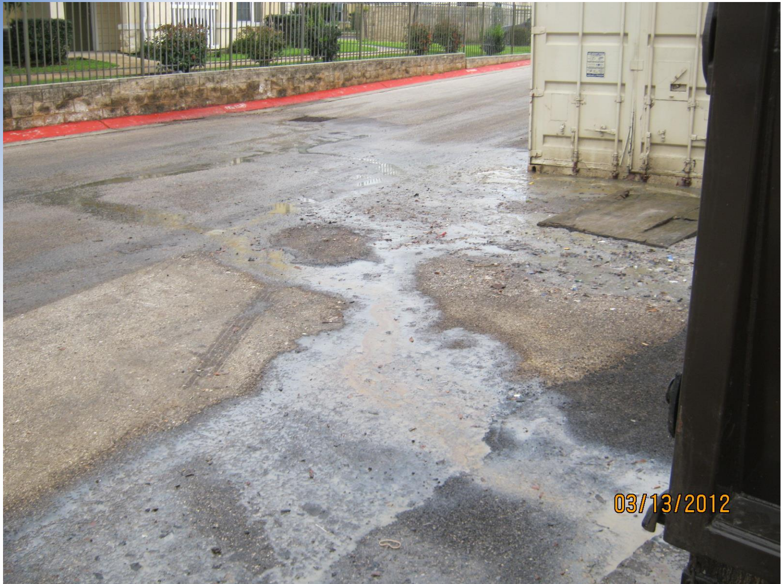
Putrescibles leaking from trash compactor.
