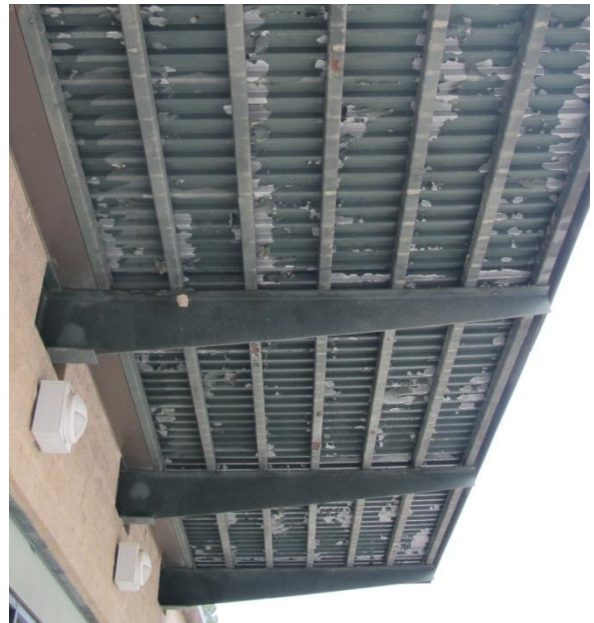
Some park and ride infrastructure requires upgrading and maintenance.
