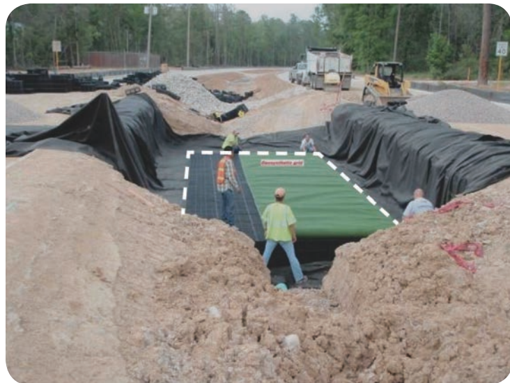
Underground storage tank, Birnamwood Drive
