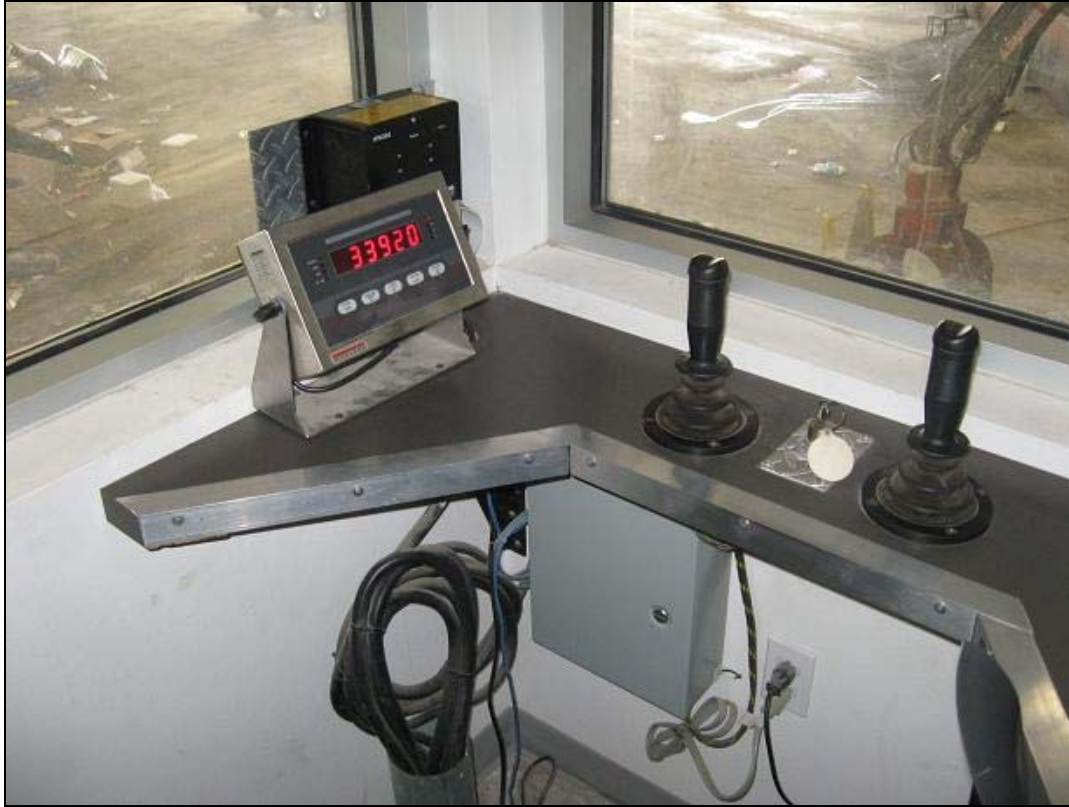
Figure 4-5. Transfer Trailer Scale Read-out and Crane Controls
