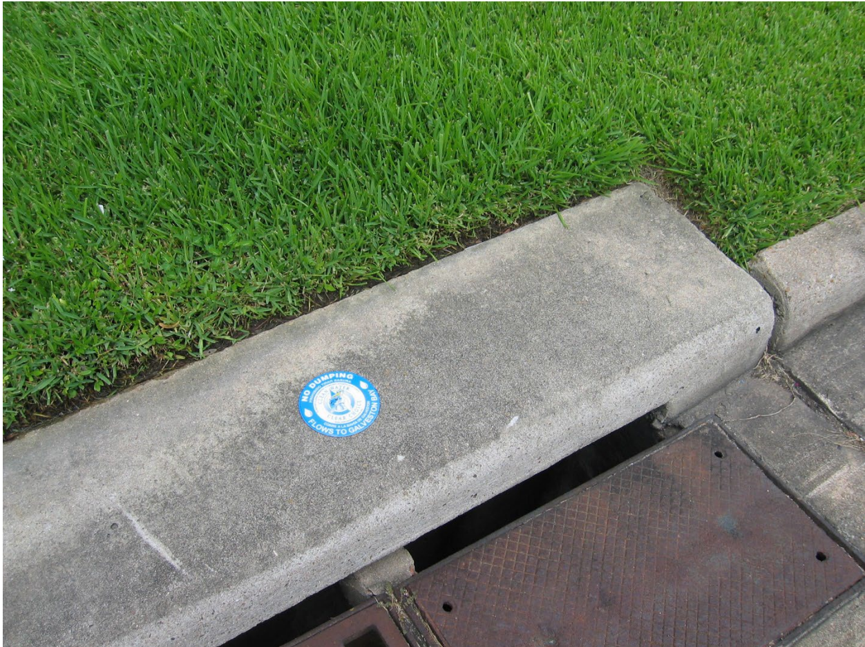
Figure 49 - Inlet marker on storm drain
