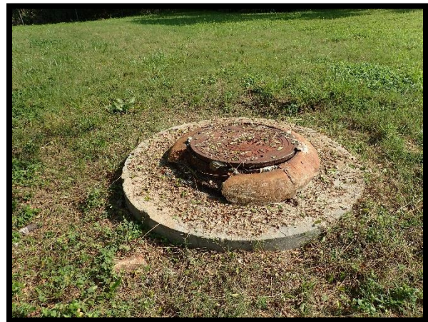
Figure 9. Aging infrastructure with evidence of sewage overflow
