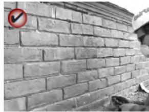
Re-point mortar joints where there is evidence of deterioration.
