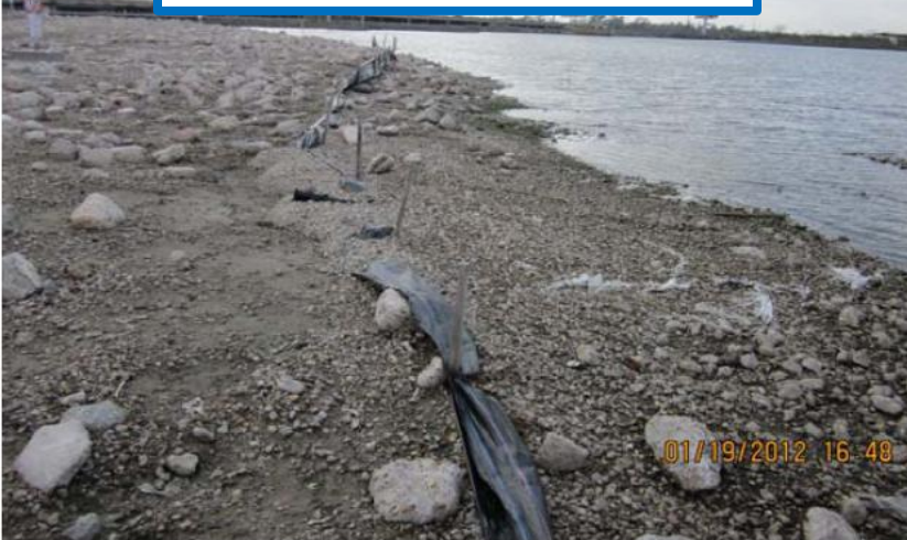
Photo: 49 Silt fencing along the northern shoreline of the Western Cell (view west)
