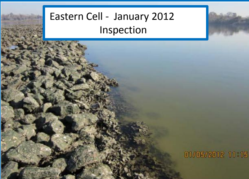
Photo: 12 View of thickened edge Eastern Cell adjacent to the San Jacinto River; photo shows intact armored cap for areas unable to be surveyed (view north)
