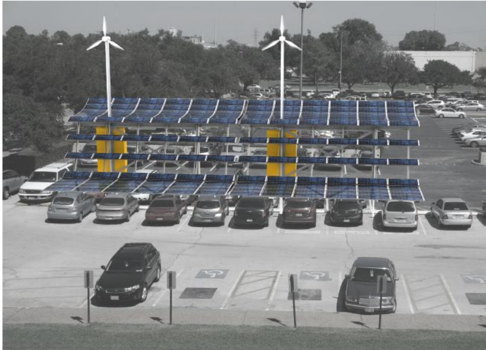
VIEW OF SOLAR PANELS AND WIND TURBINES
