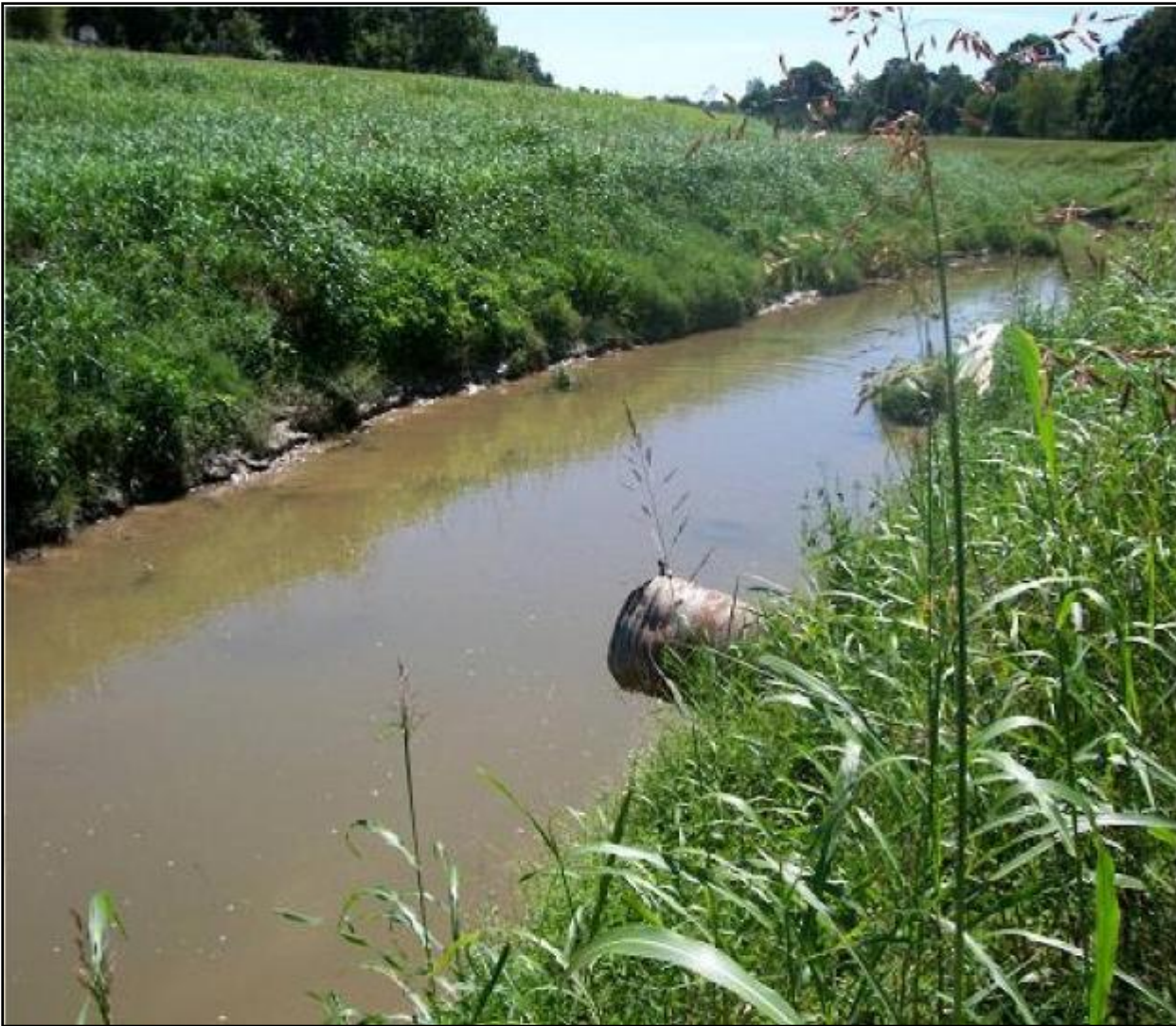
Figure 12: Westfield Estates Watershed Stormwater Outfall into Channelized Halls Bayou (Photo Source: H-GAC, 2006)
