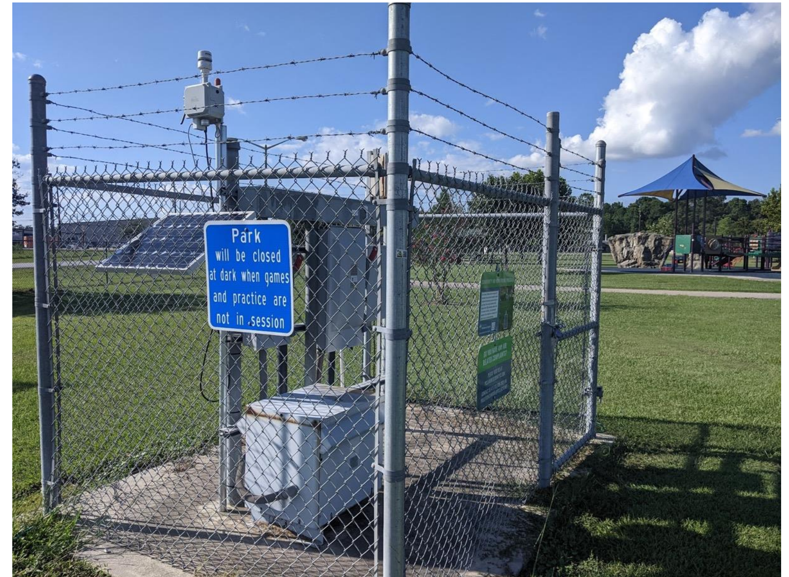
Mounted to existing utility structure in Lindsay Lyons Park
