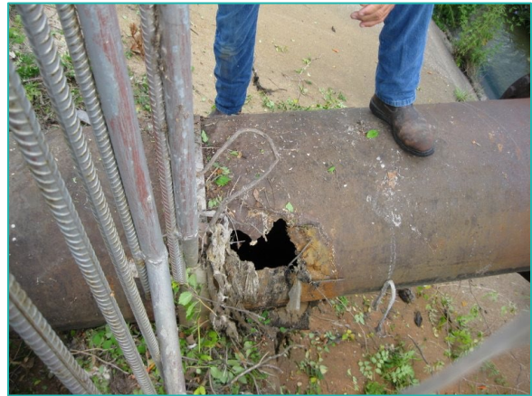
Figure 5. Broken Sanitary Sewer Line
