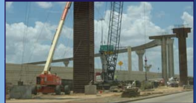
SH 99 – Work on the SH 99 Grand Parkway continues with the construction of overpasses at key at-grade intersections along Segment D. Other improvements include the construction of four direct connectors at IH-10.
