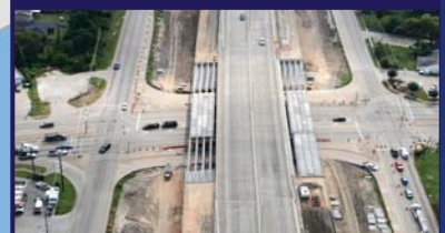
Beltway 8 – The widening of Beltway 8 from four to eight tollway lanes is a $120 million project sponsored by the Harris County Toll Road Authority (HCTRA). This project begins at US 59 and continues east to SH 288.
