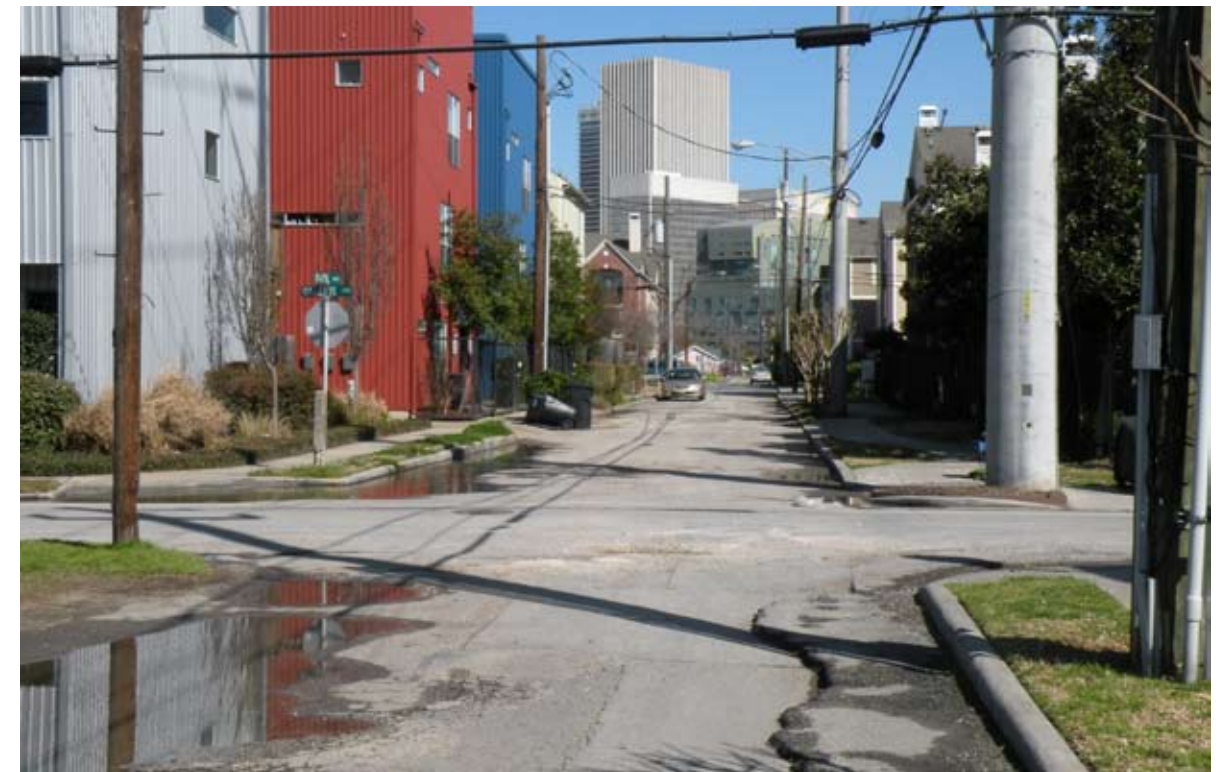
Failing and undersized storm pipes are in need of updates and replacement. A comprehensive study of the system should take place before any major construction projects are underway.
