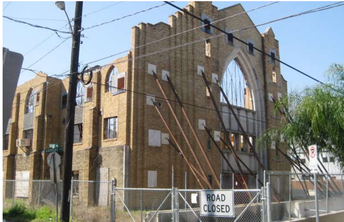
The shell of the Bethel Baptist Church is all that remains after a devastating fire in 2005. This structure is now owned by the parks department (HPARD), who is in the process of developing a park that utilizes the shell as part of the program.
