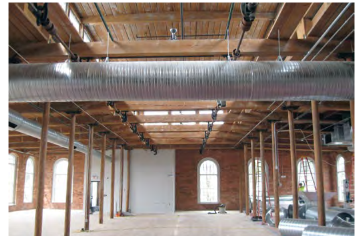
[39] Leaving the ceiling structure exposed and installing exposed ductwork where it does not impact the windows, are appropriate treatments when rehabilitating an industrial building for another use.
