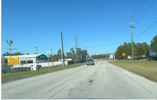
Figure 12 Airport Rd asphalt roadway with cracked pavements
